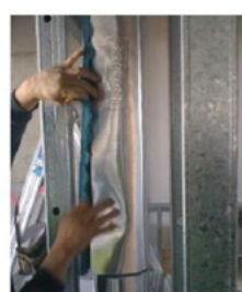
Continue lagging adjoining pipe area with the recommended overlap and joint treatment
